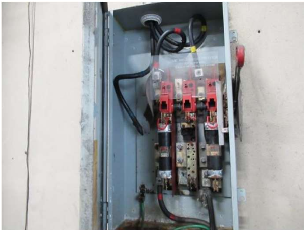
Leaking Roof – Water in Panel
