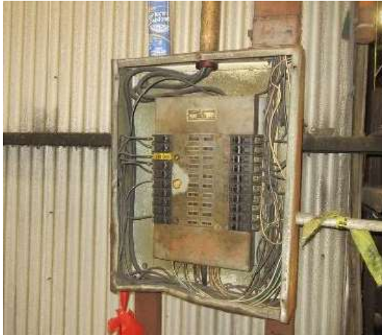
Dead front cover missing
